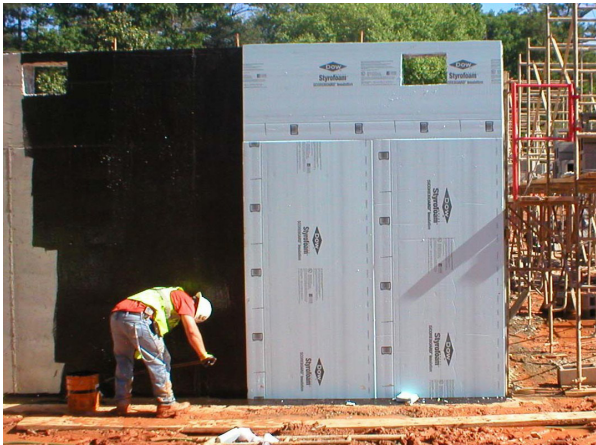
Installation of a waterproof coating installed under continuous insulation on a concrete wall.
