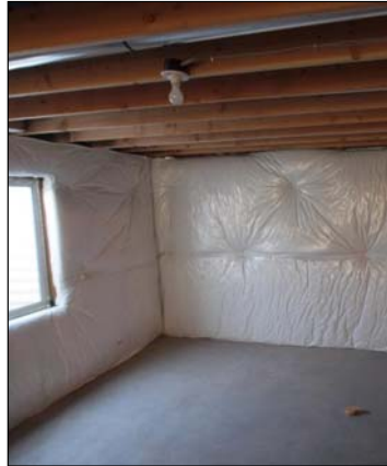
Fiberglass batt w/ vinyl backing
